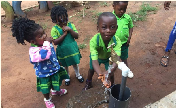
The water faucets at harvest are now connected to the bore well.
